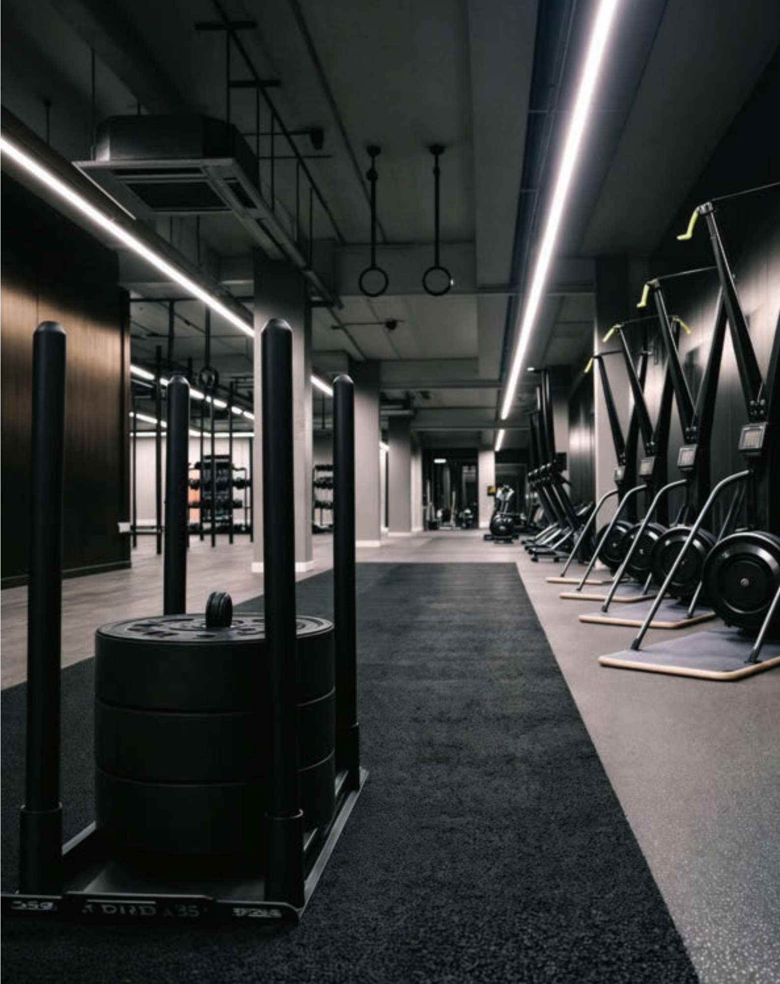
XO Fitness Gym in Ilkley Lighting design: RICOMAN Lighting. Electrical contractor: TAC Electrical
